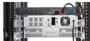
HotSwap MBPs rackmounted horizontally in rack
